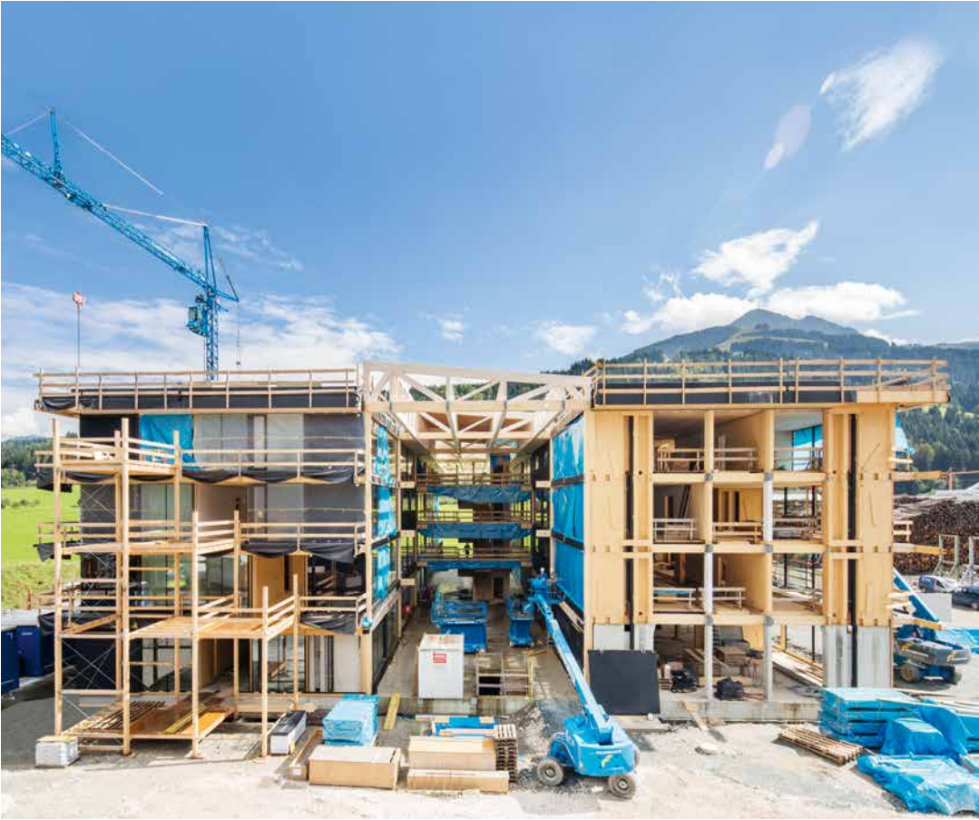
The headquarters in St. Johann in Tirol (AT) in the construction stage: The administration building made with our own materials provides space for more than 250 employees.
