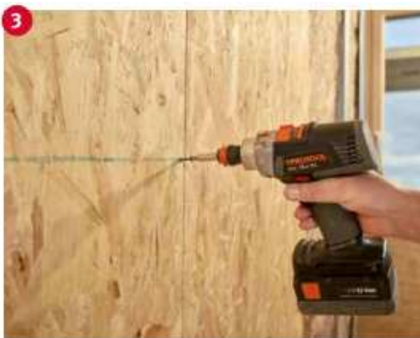
(Image 17): Fasten the first Ergo Board with a fastener spacing of 150 mm.
