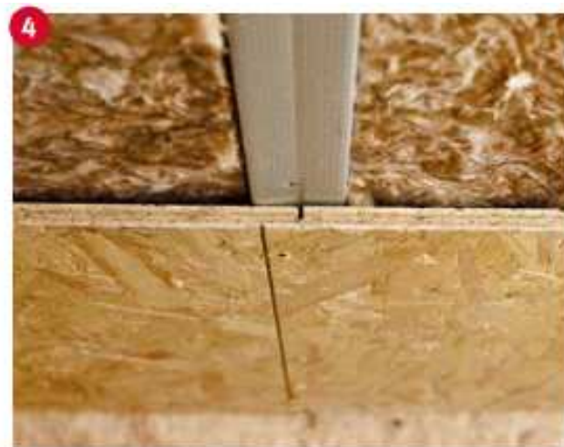
(Image 18): Fasten the upright interlocked Ergo Board panels in the step seam area with a screw into the stud frame.
