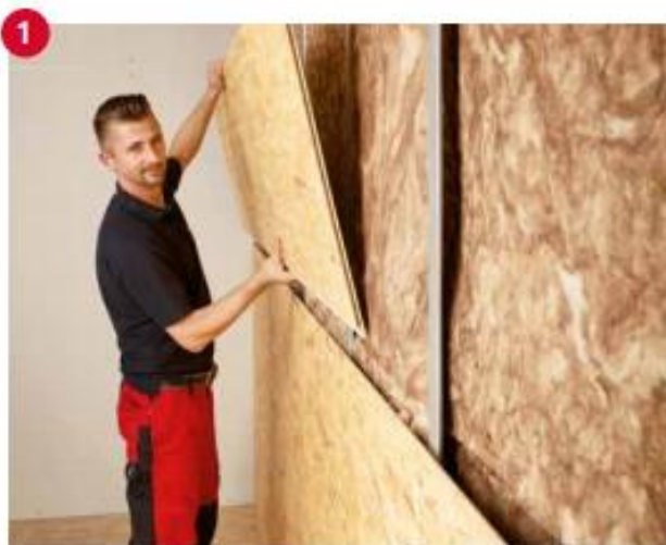
Insert the Ergo Board with the step fold on the long side. To ensure that the various edge profiles are in the correct position, the marking on the surface must be legible from left to right.
