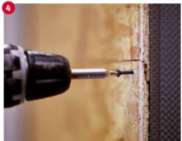
Fastening of the horizontal joints in the stand with a screw. The fastening distance at the edge of the panel is 150 mm, in the center of the panel 300 mm.
