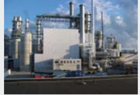
WISMAR , 1999, extension 2006. Combustion heat performance: 80 MW Steam performance: 101 t/h
