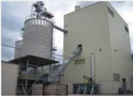
HEXHAM , since November 2007 Combustion heat performance: 50 MW 12 MW thermal oil and 38 MW hot gas current
